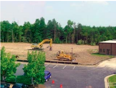
Construction at TAG, above , began in March and is expected to be completed in 2005. Below Right , Executive Vice President and Chief Operating Officer Marcus DeSouza, says the expansion will help TAG meet aggressive design and production schedules for its new military programs.
